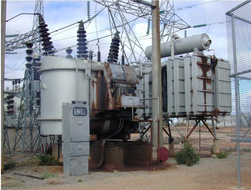
Figure 1 A transformer left in poor condition
