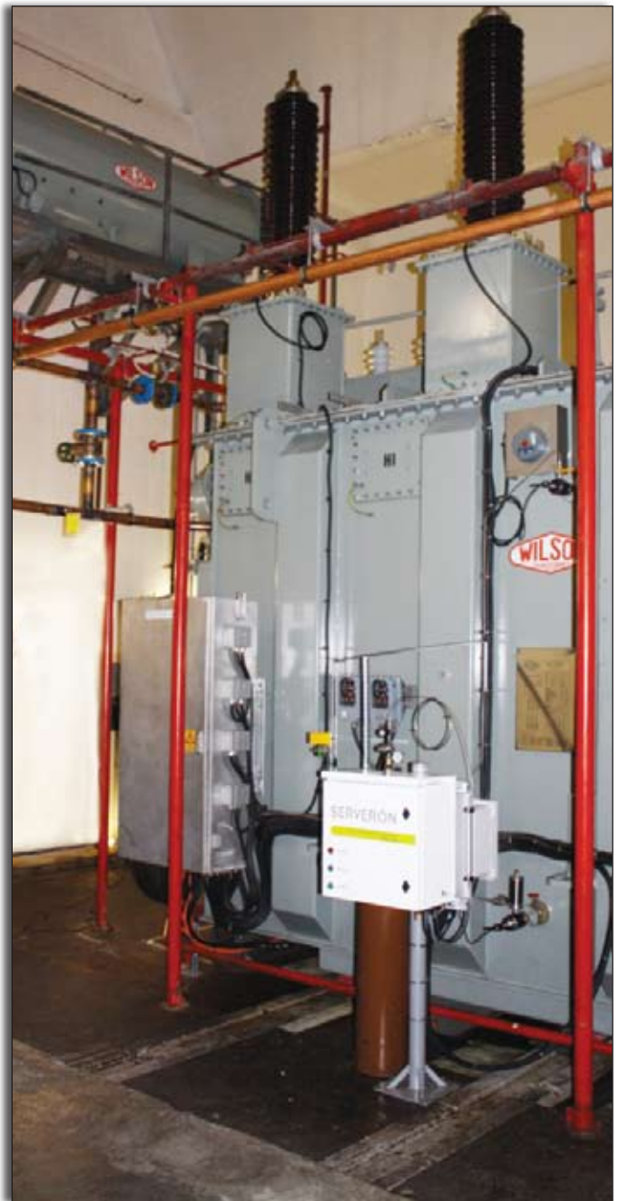
Using Envirotemp FR3 fluid in a new transformer installed in the basement of a Sydney CBD building.
